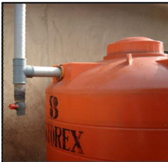
Plate 3: Tank with Pipe and Tap
