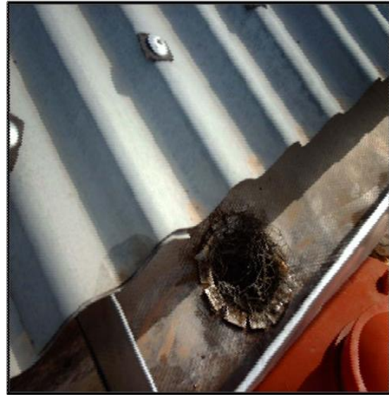
Plate 2: Gutter with Mesh
